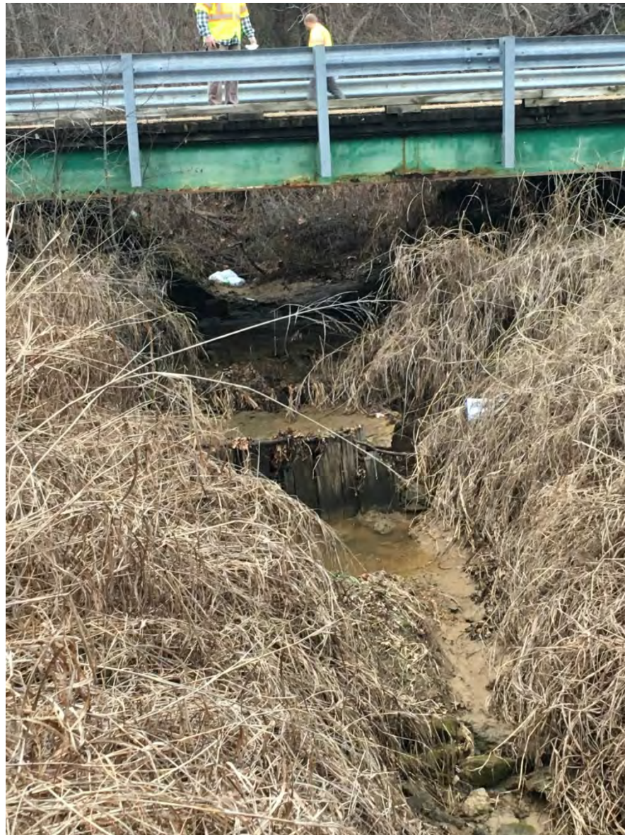
Corrosion of Girders at Outlet
