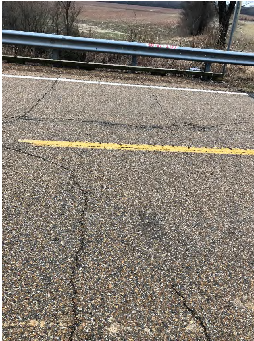
Severe Cracking on Bridge Surface
