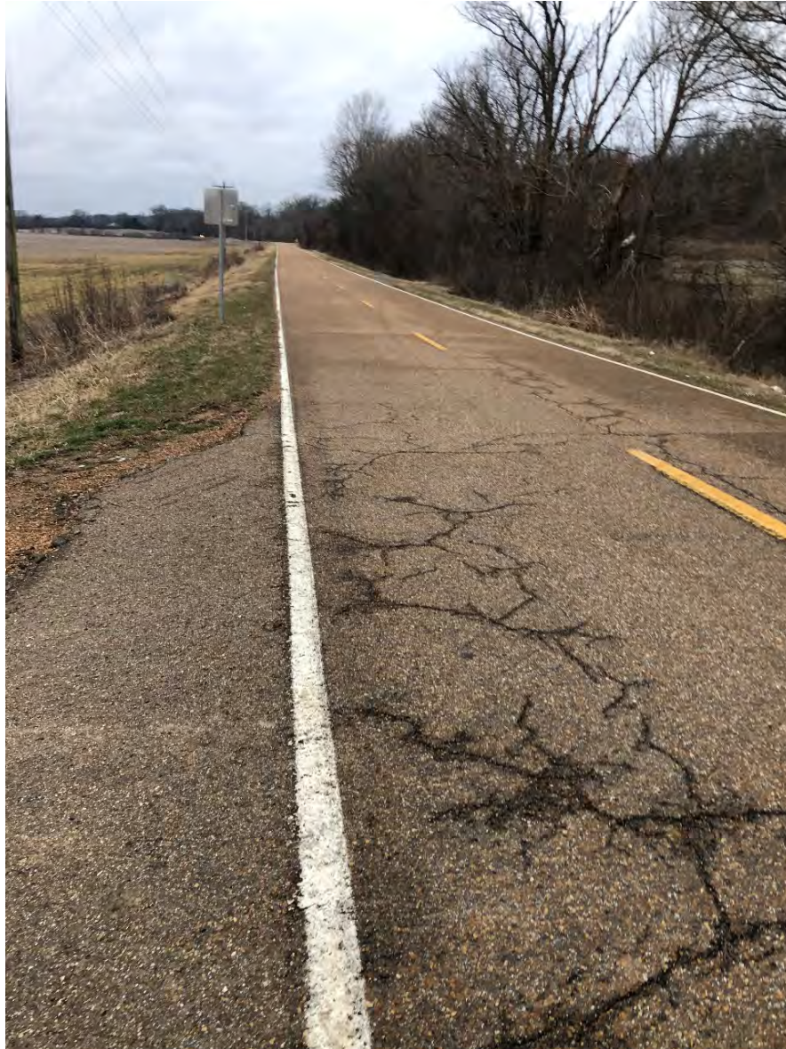
Cracking and Spalling of Pavement at West Approach
