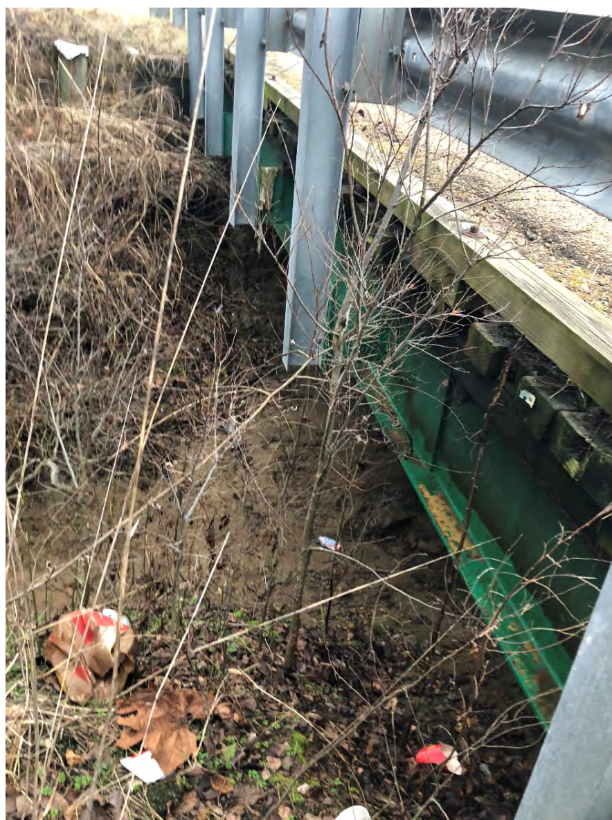
Corrosion and Vegetation of Girders at Inlet
