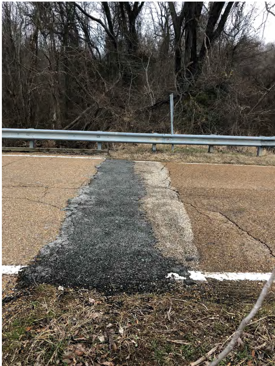
Cracking and Poor pavement patching conditions at East approach
